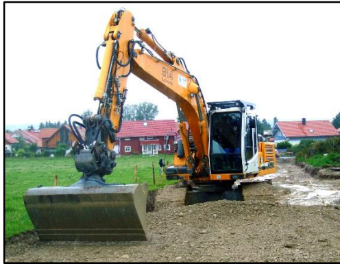
Excavator fitted with Xsite building the new street on the new Esele site in Apfeldorf
