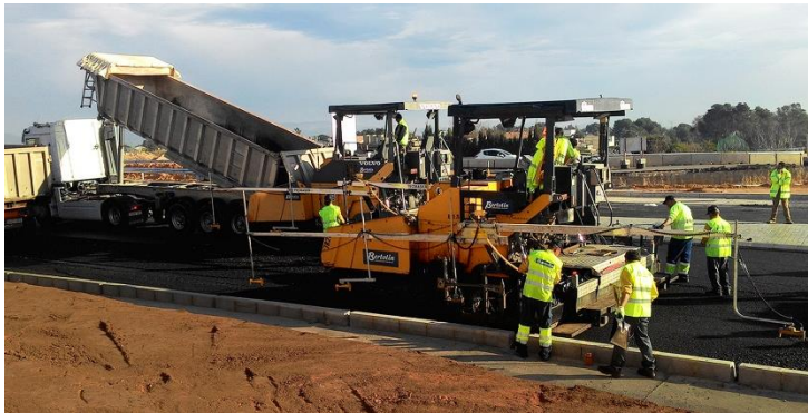
Asphalt paving during the construction of the new CV-370 in the province of Valencia
